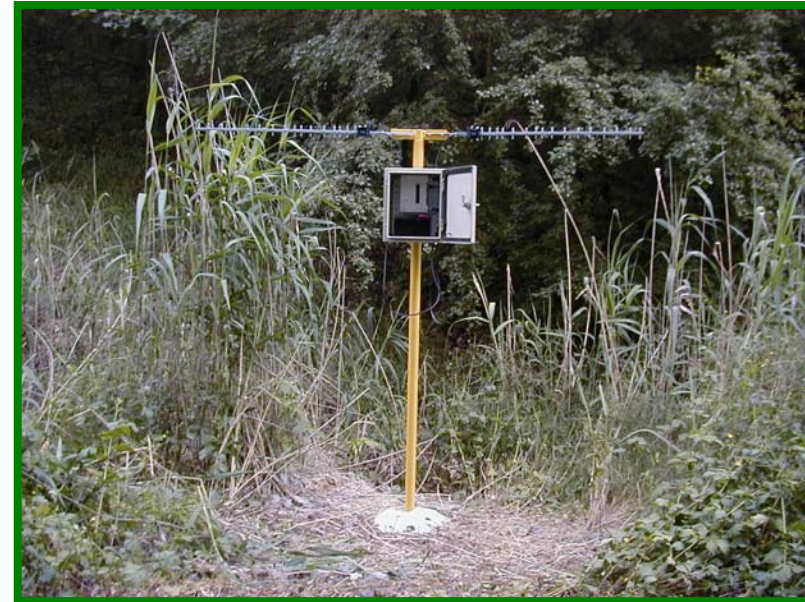
2.4 GHz CDMA repeater. The wireless LAN installed along the trial track enables remote control of the mobile robots on the 4 km long trial track in Pardubice station.
